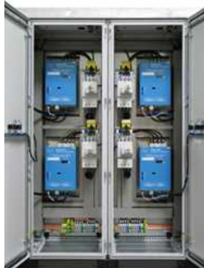
Fig. 12-5 Control cabinet with four inverters
