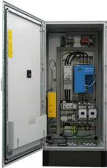
Fig. 12-4 Control cabinet with electrode holder changeover
