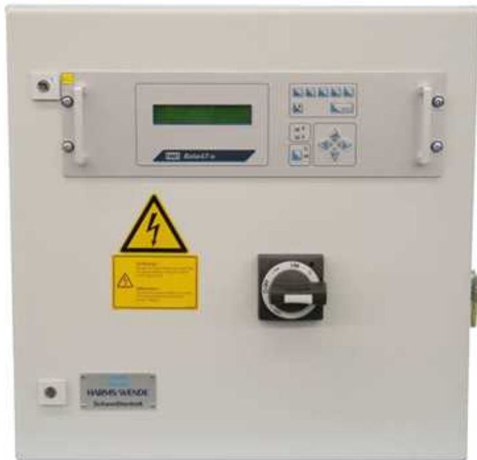
Fig. 10-3 MPK43 control cabinet
